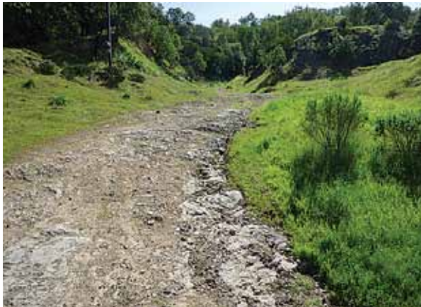
Figure 3.22 Competent shallow bedrock can minimize the amount of erosion, but at the same time can lead to an uneven road/trail surface.
