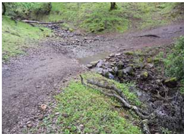
Figure 3.41 Rock ford on unsurfaced road. Ford constructed using native rock to armor outer road edge.
