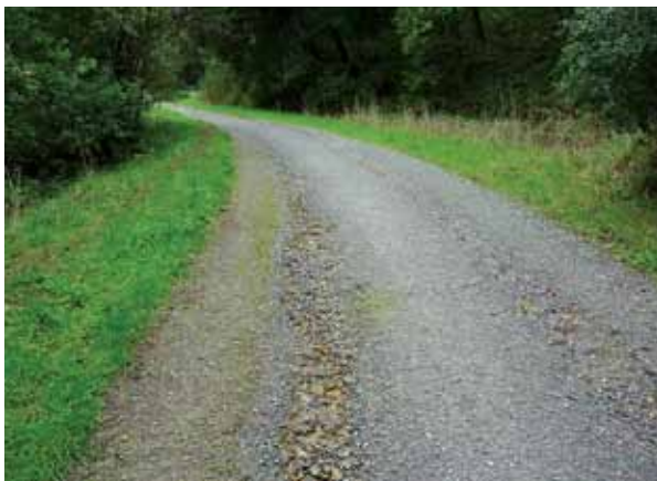
Figure 3.18 Erosion on rocked road attributed to lack of cross drains. Vehicular use of the road has resulted in shallow rutting along the wheel tracks.
