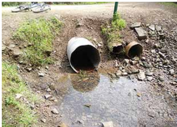
Figure 3.39 Stream crossing with culvert. Note the two smaller pipes, which were undersized and became plugged with sediment.
