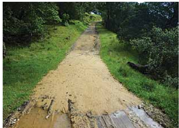
Figure 3.19 Sediment from erosion of the road bed is deposited in a natural dip. Frequently placed drainage dips could have minimized this erosion.
