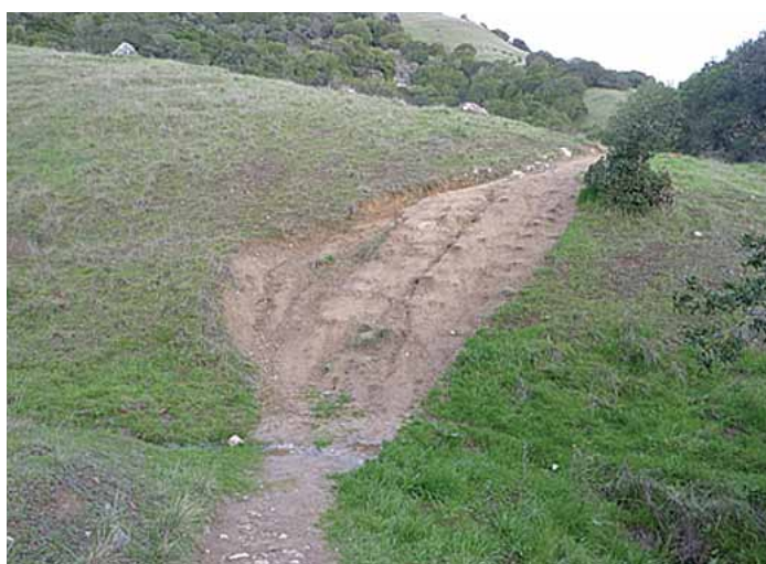
Figure 3.12 The lower Vogelsang Trail was widened as a result of visitor use. This steep fall line segment of trail drains to a watercourse at the base of the hillside.
