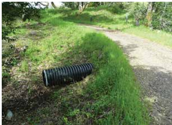
Figure 3.40 Recently installed plastic pipe. Outlet is "shotgunned," leading to erosion at the outfall.
