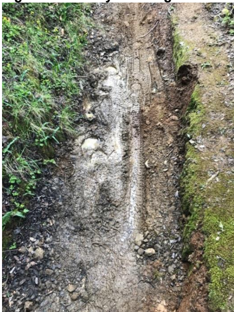
Figure 10: Poorly Draining Trail
