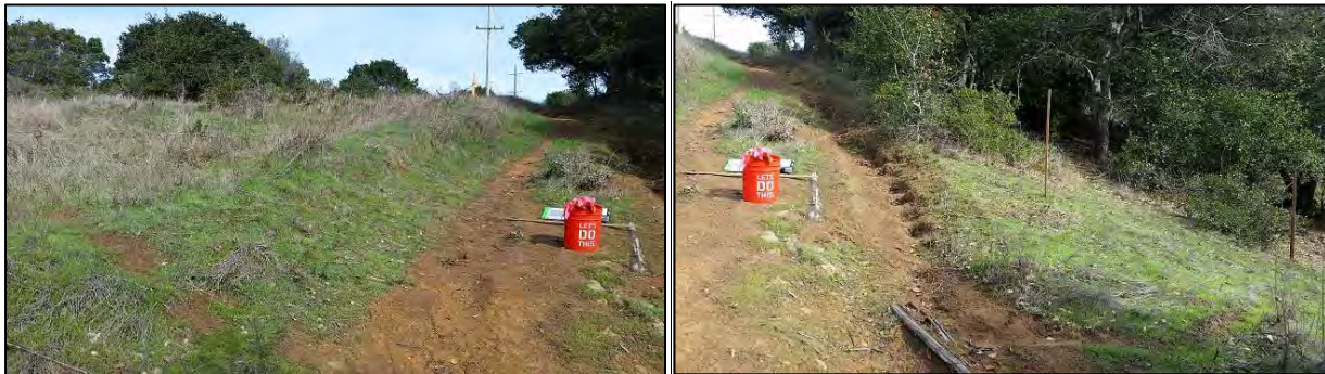
View upslope along lower portion of existing Gas Line Trail, in vicinity of field-measured topographic profile at Waypoint 28 (see Figure 4 for waypoint location, Figure 6 for topographic profile). Berm over gas line visible at left; gullied area exposes deeply weathered rock.
