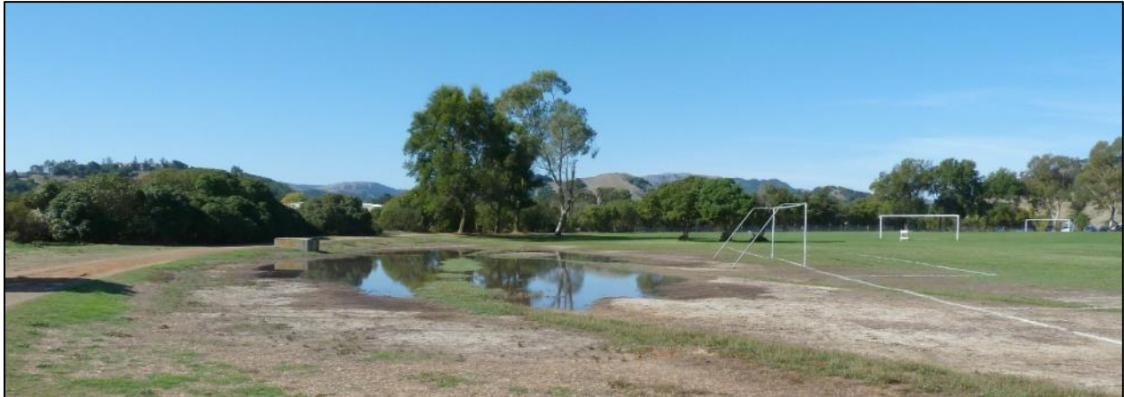
Figure 2-19: Surface Ponding at McInnis Soccer Field
