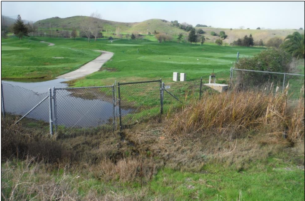
Figure 2-20: Surface Ponding at McInnis Golf Course Levee Crest Elevations
