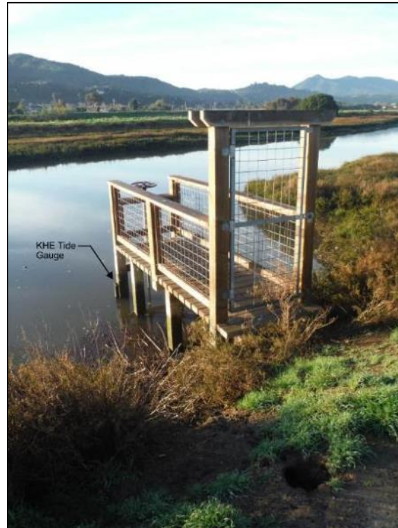
Figure 2-29: Photo of McInnis Marsh Tide Gate (TG-1) and KHE tidal monitoring stilling well (2/11/15).
